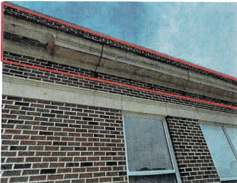
JM Hill School: Addition – Existing EIFS finish delaminated from cornice. Existing EIFS finish at cornice and frieze cracked and joints in need of repair.
