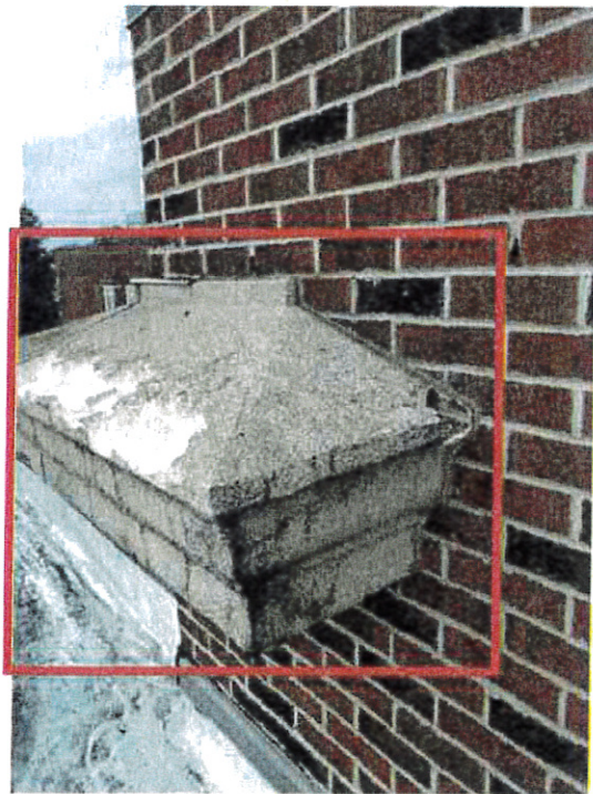
JM Hill School: Addition – Existing EIFS finish delaminated from cornice.
