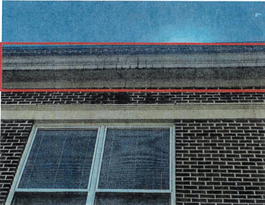
JM Hill School: Addition – Existing EIFS finish delaminated from cornice. Existing EIFS finish at cornice and frieze cracked and joints in need of repair.
