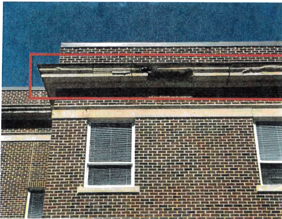
JM Hill School: Addition – Existing EIFS finish delaminated from cornice. Existing EIFS finish at cornice and frieze cracked and joints in need of repair.
