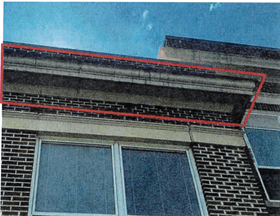
JM Hill School: Addition – Existing EIFS finish delaminated from cornice. Existing EIFS finish at cornice and frieze cracked and joints in need of repair.
