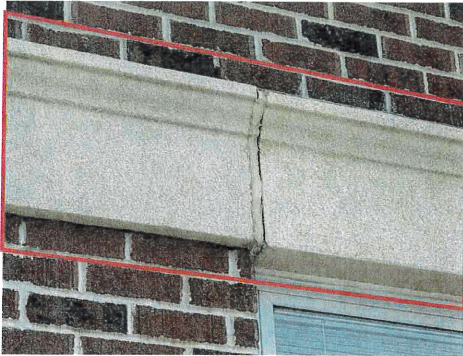
JM Hill School: Addition – Existing EIFS finish at frieze cracked and joints in need of repair.
