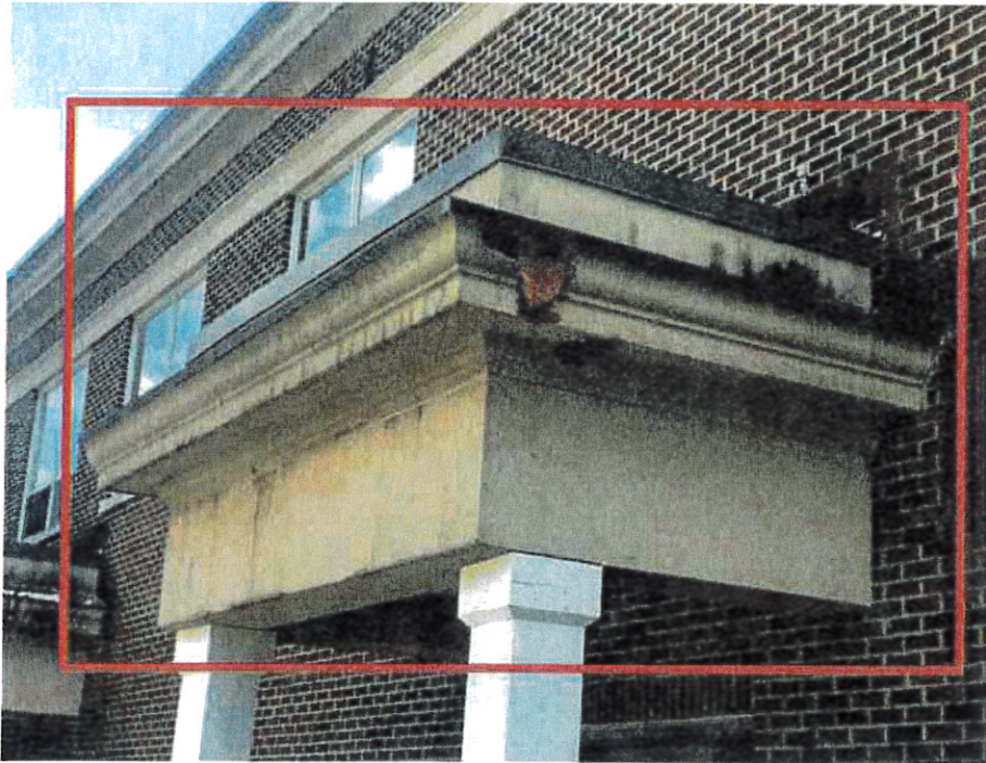
JM Hill School: Addition – Existing EIFS finish delaminated from cornice. Existing EIFS finish at cornice cracked and joints in need of repair.
