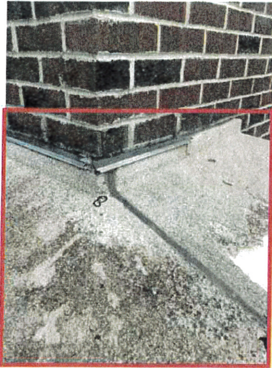
JM Hill School: Addition – Existing EIFS finish delaminated from cornice. Existing through wall flashing in need of repair.
