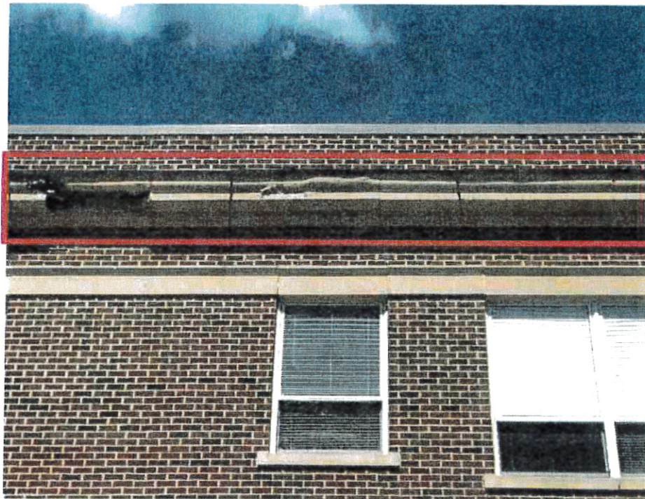
JM Hill School: Addition – Existing EIFS finish delaminated from cornice. Existing EIFS finish at cornice and frieze cracked and joints in need of repair.
