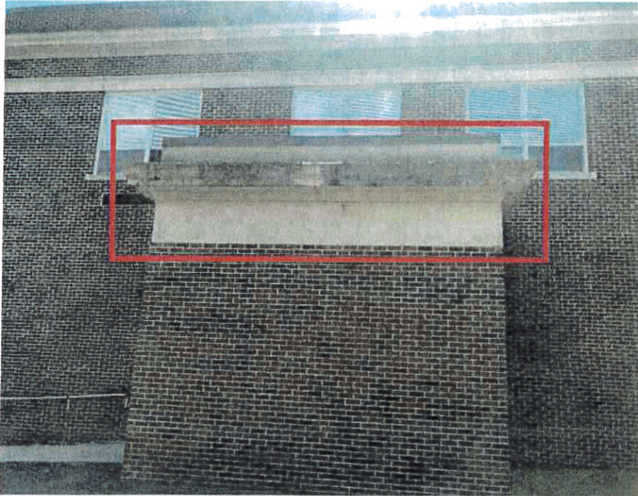
JM Hill School: Addition – Existing EIFS finish delaminated from cornice. Existing EIFS finish at cornice cracked and joints in need of repair.
