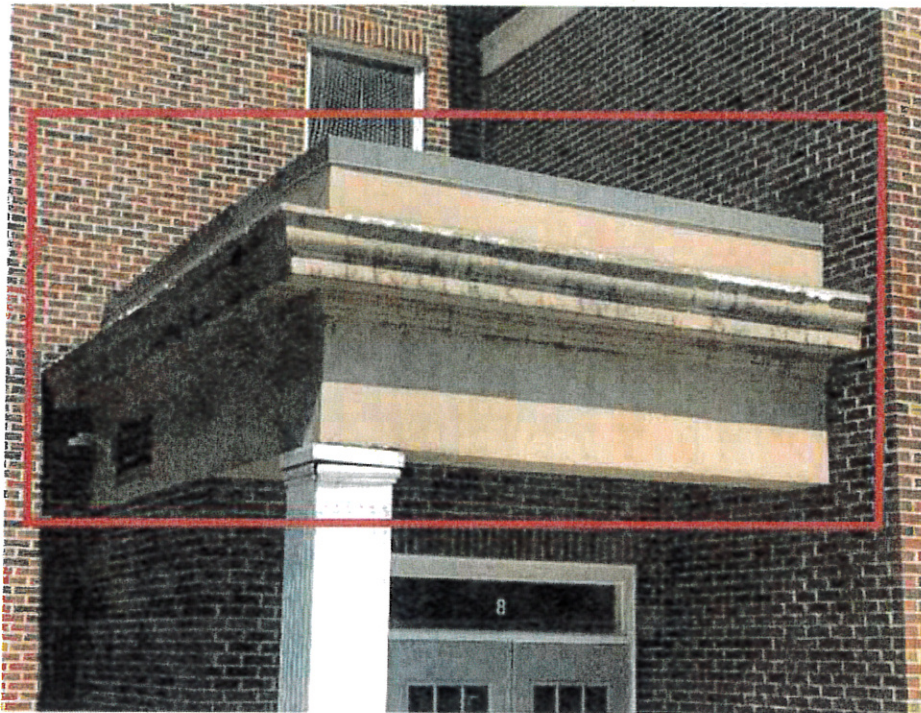
JM Hill School: Addition – Existing EIFS finish delaminated from cornice. Existing EIFS finish at cornice cracked and joints in need of repair
