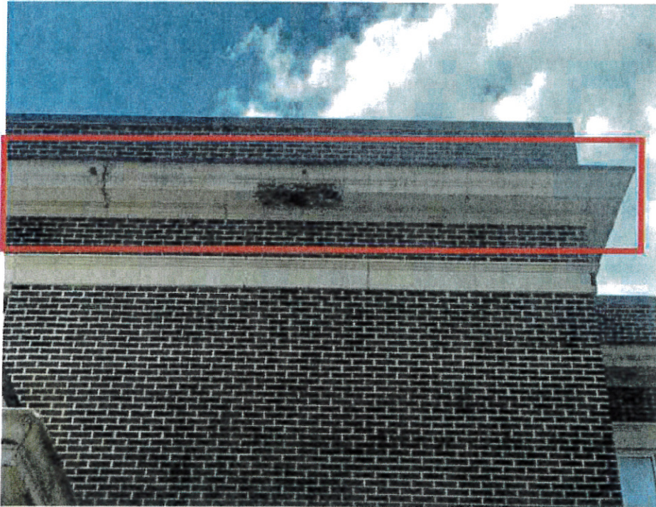
JM Hill School: Addition – Existing EIFS finish delaminated from cornice. Existing EIFS finish at cornice and frieze cracked and joints in need of repair.
