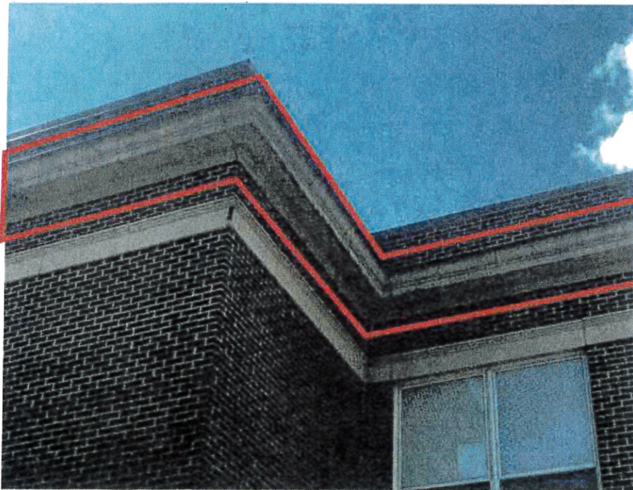
JM Hill School: Addition – Existing EIFS finish delaminated from cornice. Existing EIFS finish at cornice and frieze cracked and joints in need of repair.
