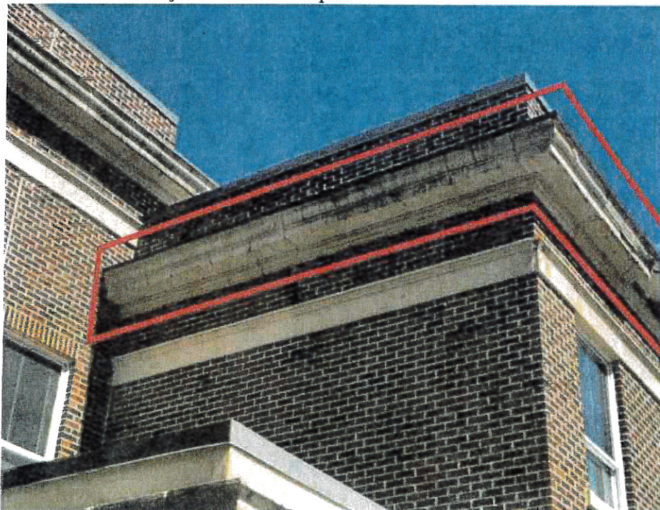
JM Hill School: Addition – Existing EIFS finish delaminated from cornice. Existing EIFS finish at cornice and frieze cracked and joints in need of repair.
