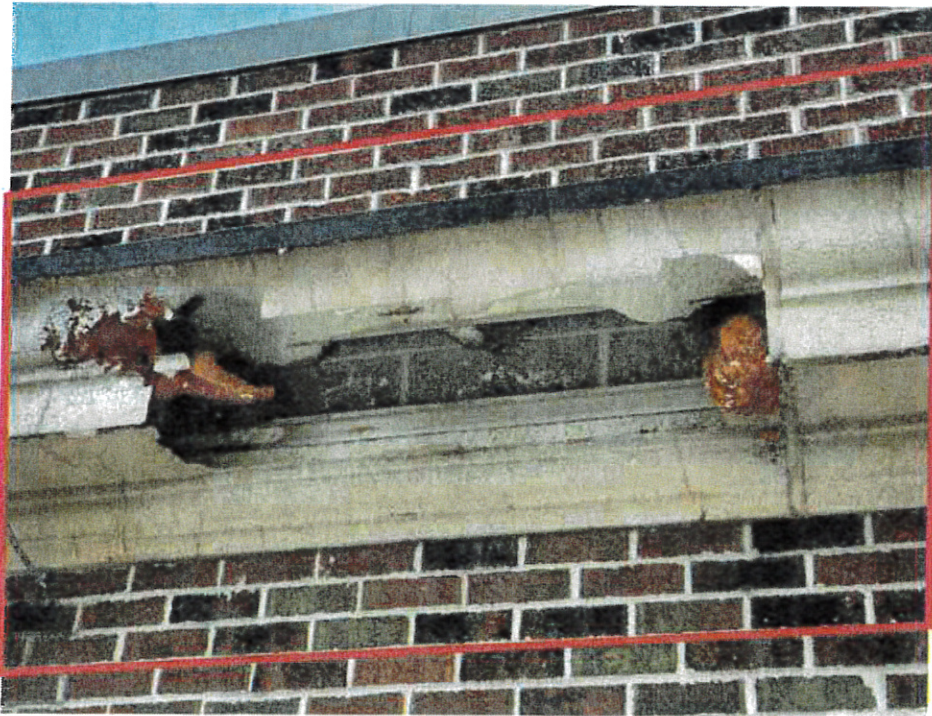
JM Hill School: Addition – Existing EIFS finish delaminated from cornice.
