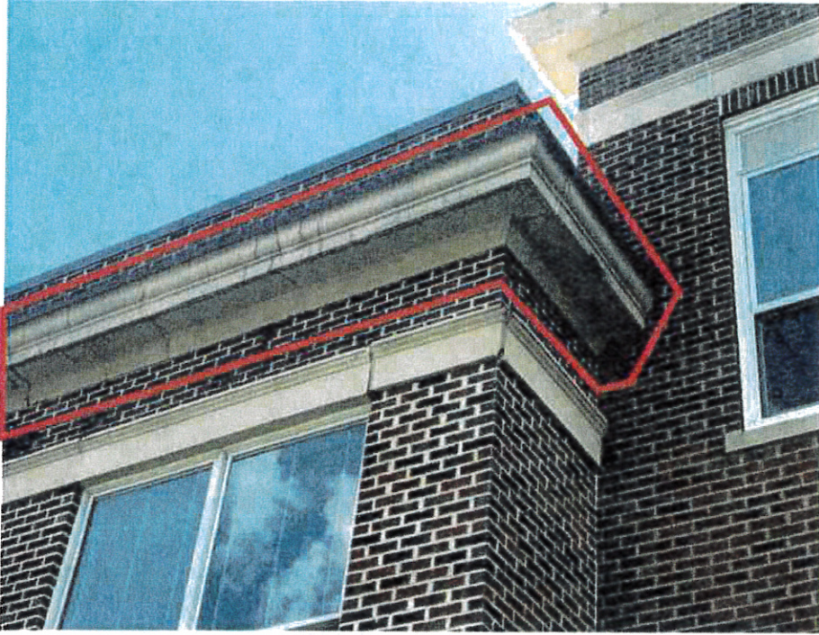
JM Hill School: Addition – Existing EIFS finish delaminated from cornice. Existing EIFS finish at cornice and frieze cracked and joints in need of repair.
