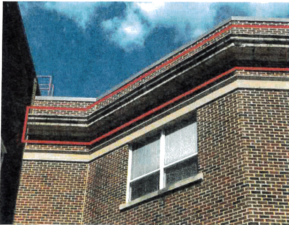
JM Hill School: Addition – Existing EIFS finish delaminated from cornice. Existing EIFS finish at cornice and frieze cracked and joints in need of repair.
