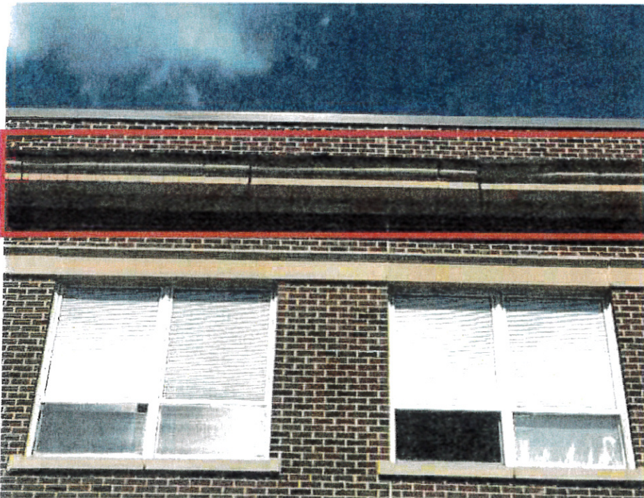
JM Hill School: Addition – Existing EIFS finish delaminated from cornice. Existing EIFS finish at cornice and frieze cracked and joints in need of repair.
