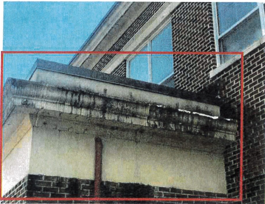
JM Hill School: Addition – Existing EIFS finish delaminated from cornice. Existing EIFS finish at cornice cracked and joints in need of repair.
