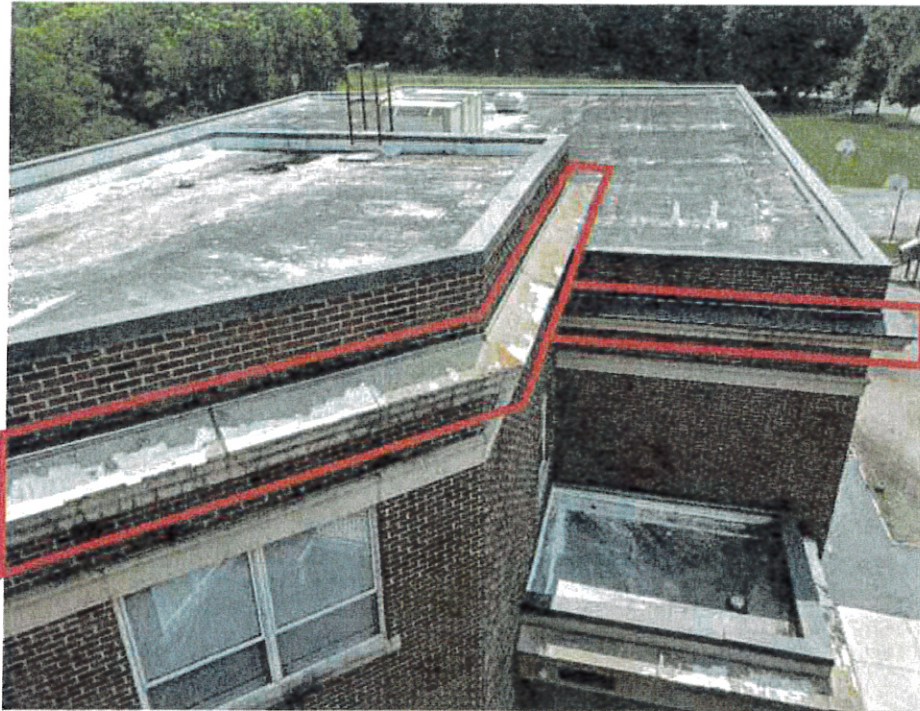
JM Hill School: Addition – Existing EIFS finish delaminated from cornice. Existing EIFS finish at cornice and frieze cracked and joints in need of repair.
