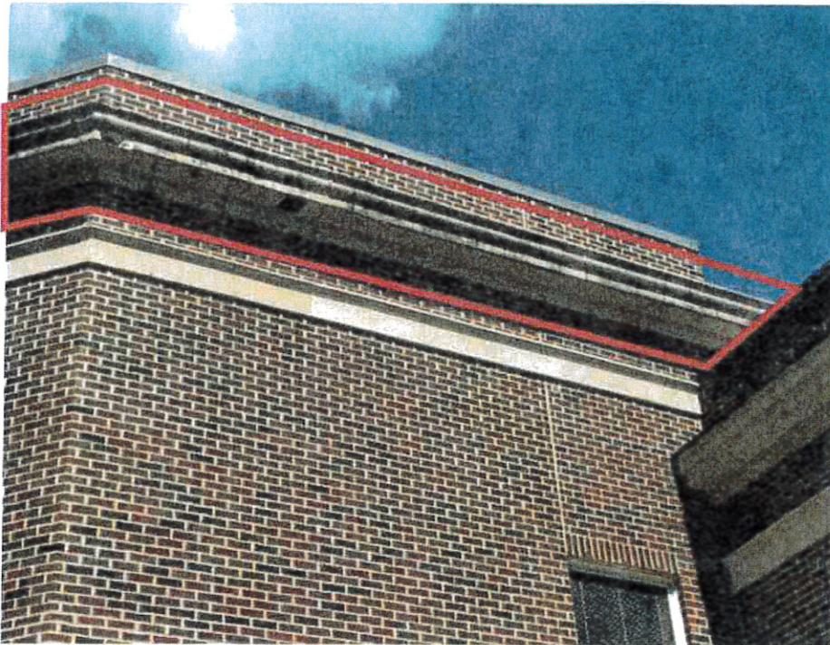
JM Hill School: Addition – Existing EIFS finish delaminated from cornice. Existing EIFS finish at cornice and frieze cracked and joints in need of repair.
