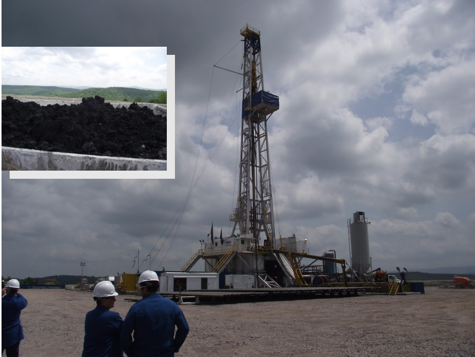
Gas drilling rig in Bradford County, Pennsylvania. Inset: Shale rock cuttings from the drilling process. Their dark color indicates a higher percentage of organic compounds contained in the shale. Shale rock with less organic content is lighter in color.
